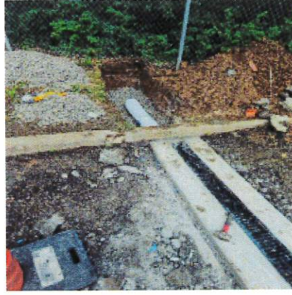
Trench drain and gravel detention
