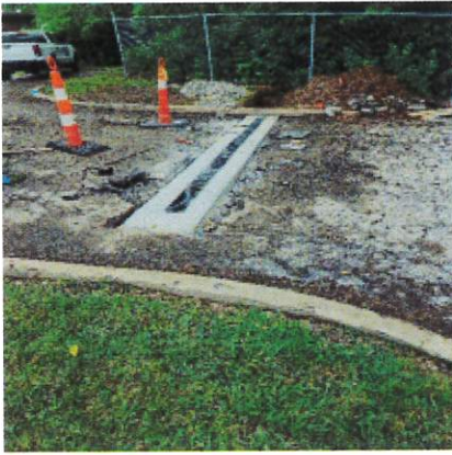
Drive entry trench drain
